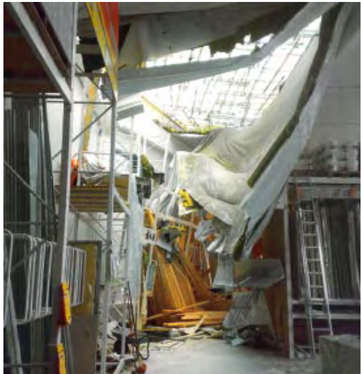
On 1 June 2008, the roof of a DIY market collapsed in Schwarzenberg (Saxony).
